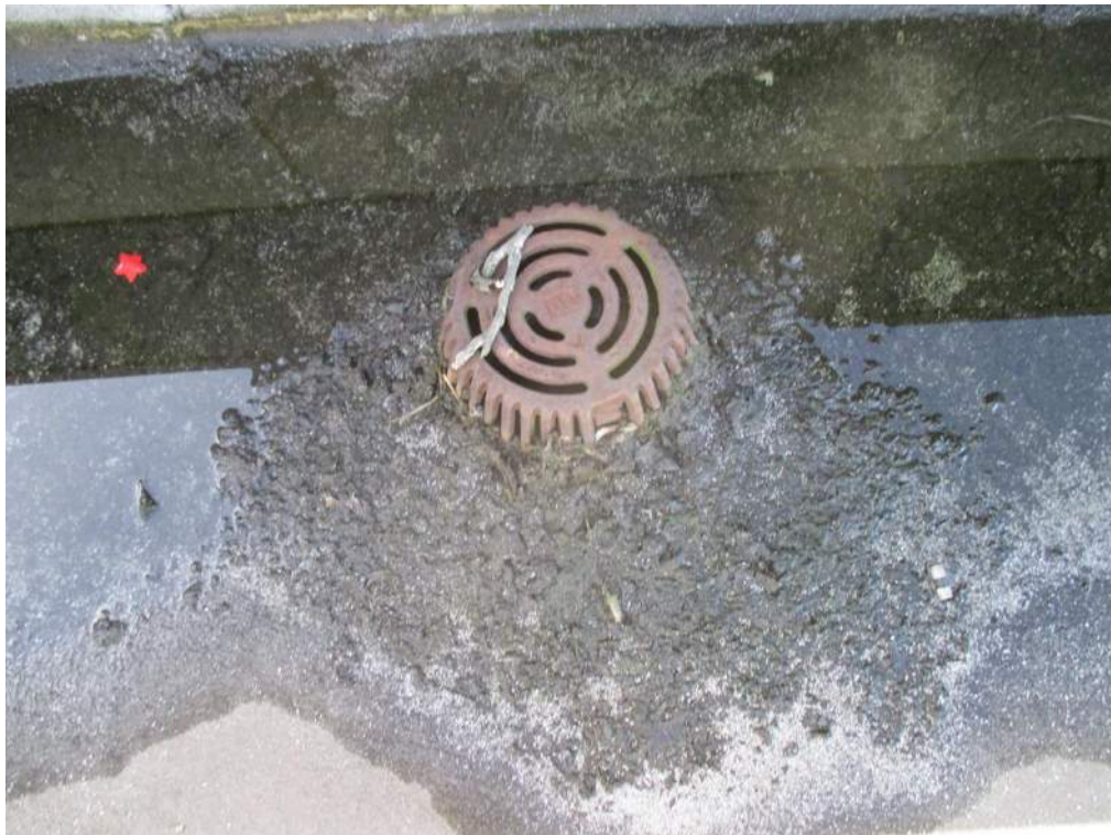
Photo 6 Clogged roof drain
