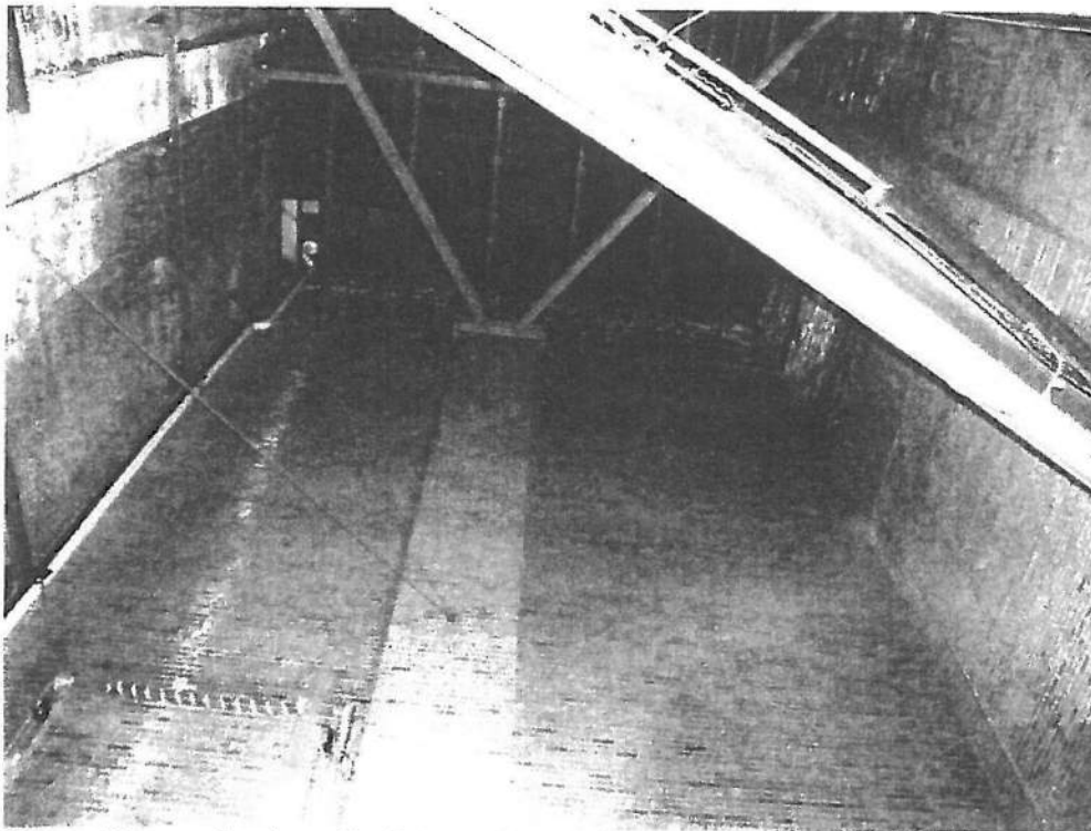
Photo 48 South wall of stage viewed from inside stage left. Proscenium wall to the right. The rear (east) wall to the left. Additional bracing is seen at the top. Efflorescence in masonry is conspicuous.
