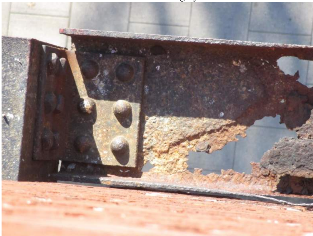
Photo 12 Steel Lateral Bracing System: Holes in the web of I beam
