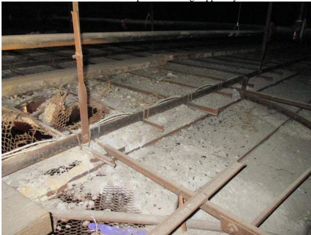
Photo 4 Damaged area of suspended ceiling.
