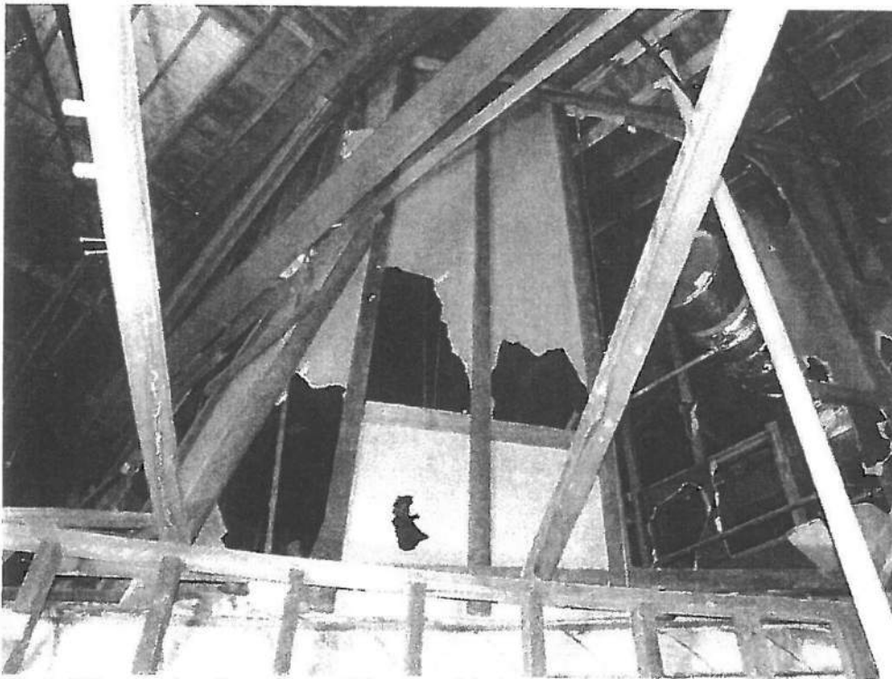
Photo 38 Another view of the metal lath and plaster ceiling from plenum along north wall. A wood stud wall has been constructed to brace the ceiling construction.
