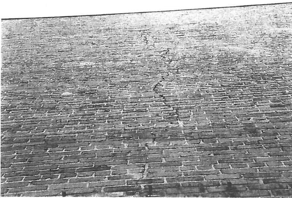
Photo 54 Close up of typical vertical crack. See attached drawings for vertical crack locations. Cracking should be repaired.
