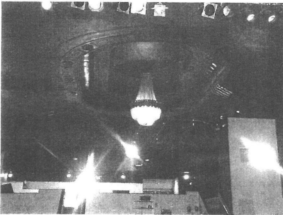
Photo 12 View of the plaster ceiling. (Viewed from downstage) Black Box theater is towards the rear.
