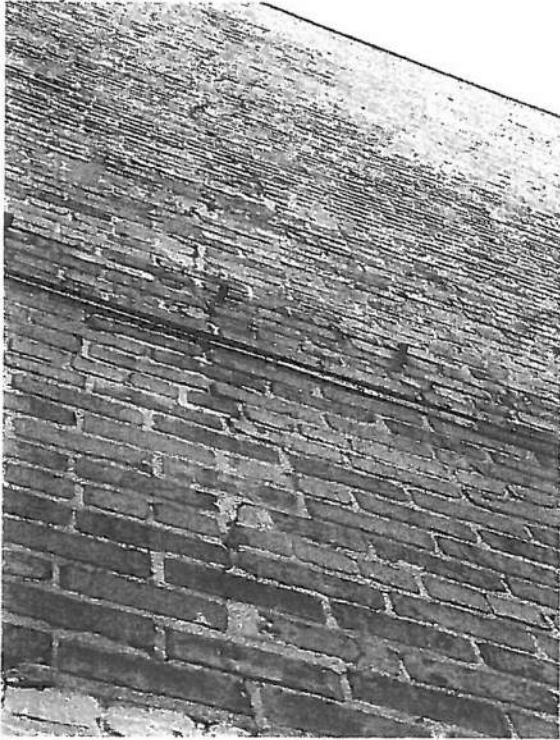
Photo 53 Close up of brick masonry with loose mortar. Conditions should be repaired.
