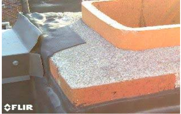
PHOTO 8 Lower Roof Section: Metal cap over chimney wash is recommended be installed and lapped over metal coping cap.
