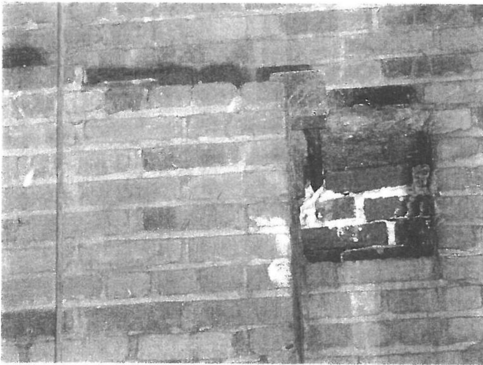
Photo 40 Missing brick and incorrect repair to wall stage right. Condition must be mitigated.
