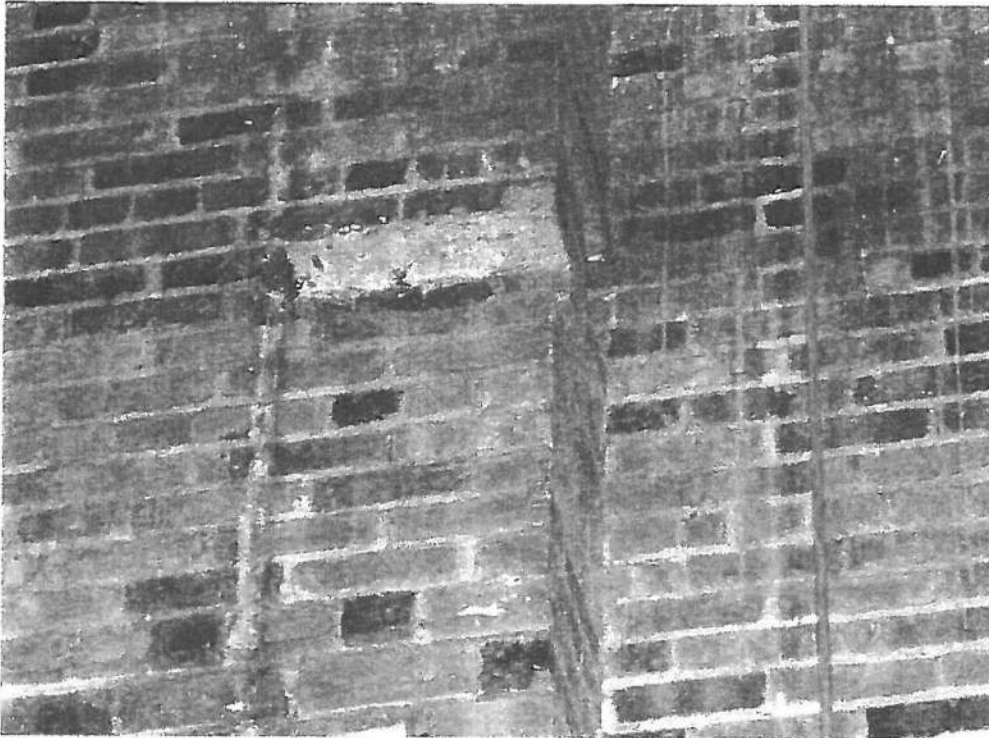
Photo 39 Missing brick in pilaster at stage right. Condition should be mitigated.
