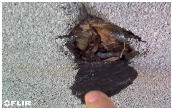
PHOTO 6 Lower Roof Section: Hole in wall flashing. Patch repair needed.
