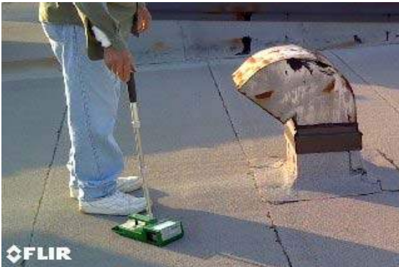
PHOTO 3 Lower Roof Section: Tramex meter was place on roof surface every 2-4 feet in grid pattern.
