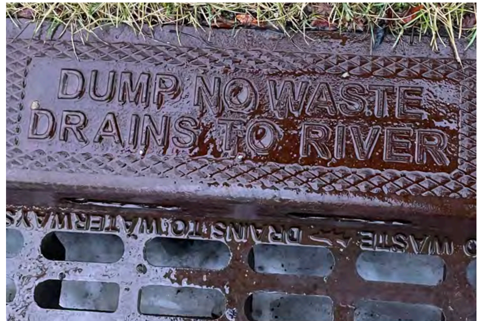
Storm Drain. Source: Colliers Engineering & Design
